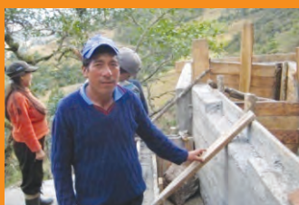
CESAR HUAMAN, LOCAL CHORRO BLANCO RESIDENT, HELPING TO BUILD THE MICRO HYDRO POWER HOUSE
