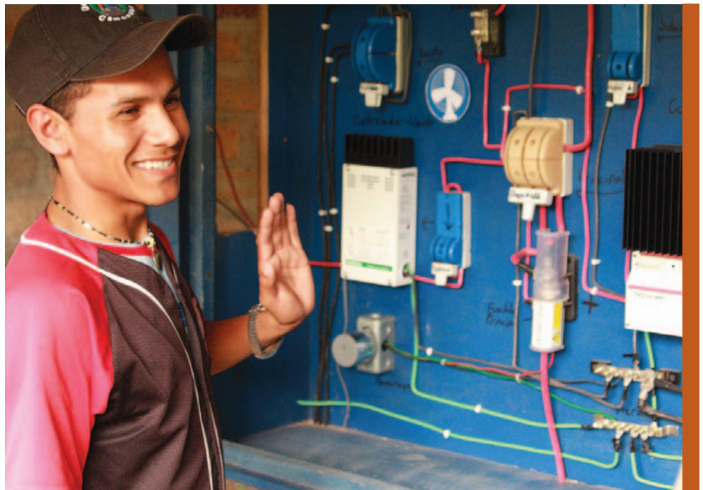
Dahley explaining how the control centre works
