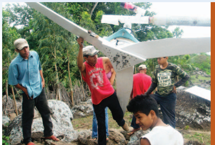
Members of the community helping to set up the wind turbine in Cajiniquil
