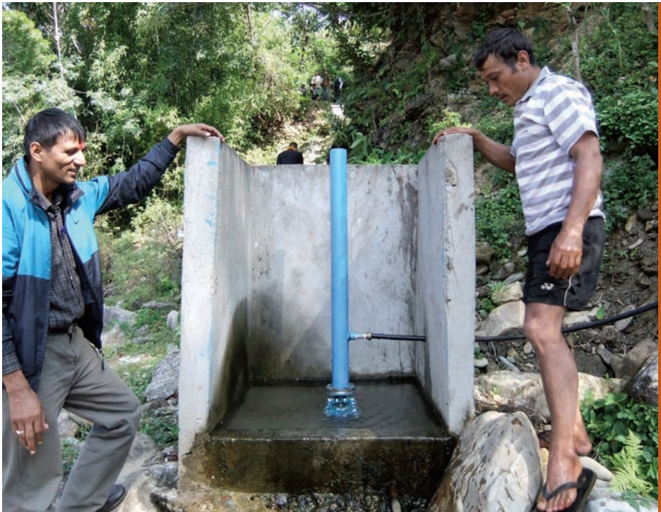
Mr Tara Bahadur Adhikari – the technician who maintains the Sunaula bazaar ram pump
